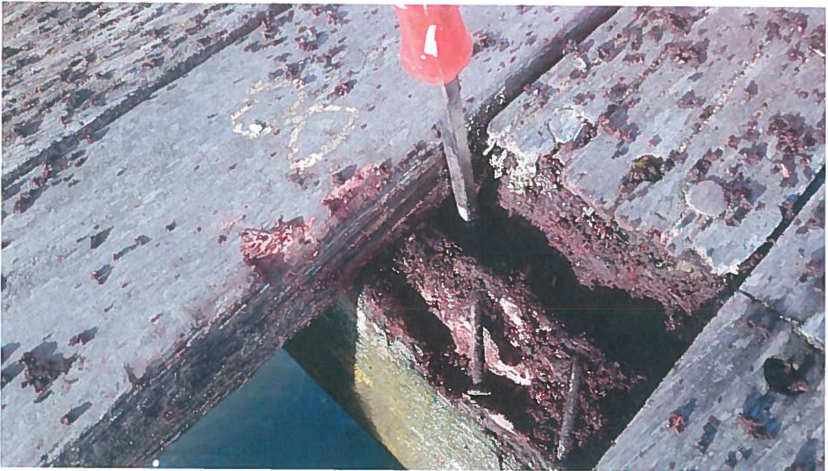
Photo 5 Joist 8 with significant loss. Stress estimated = 0.997
