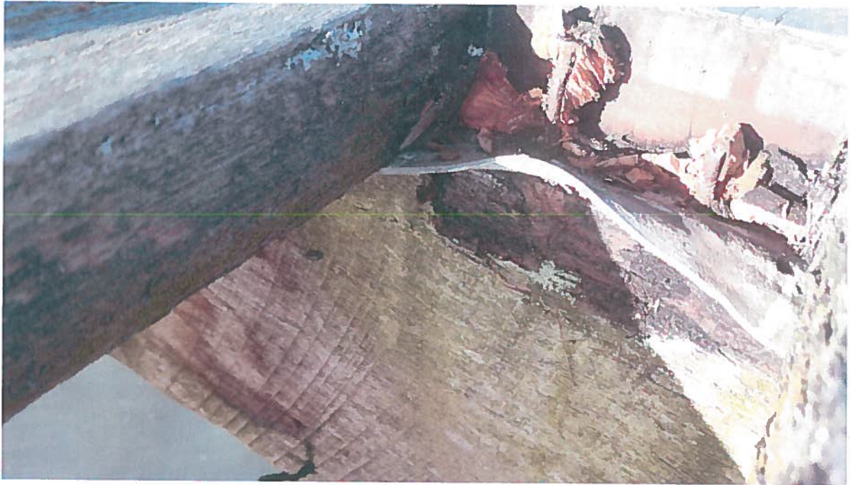
Photo 2 Joist with lead sheet over and some defective timber
