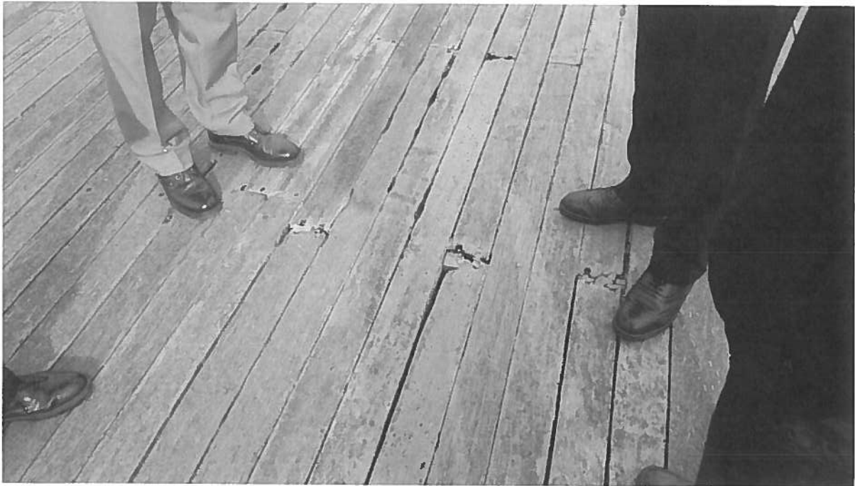
Photo 1 Deck condition typically poor at plank ends, with repairs, traps, and potential trip hazards
